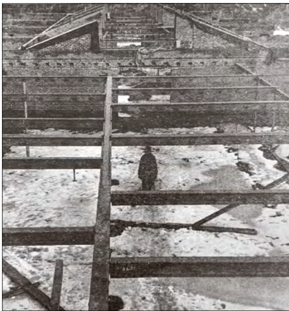
The Growing Dream...Salisbury’s new school, planned and hoped for for more than seven years, begins to take on a three-dimensional reality of brick and steel.
