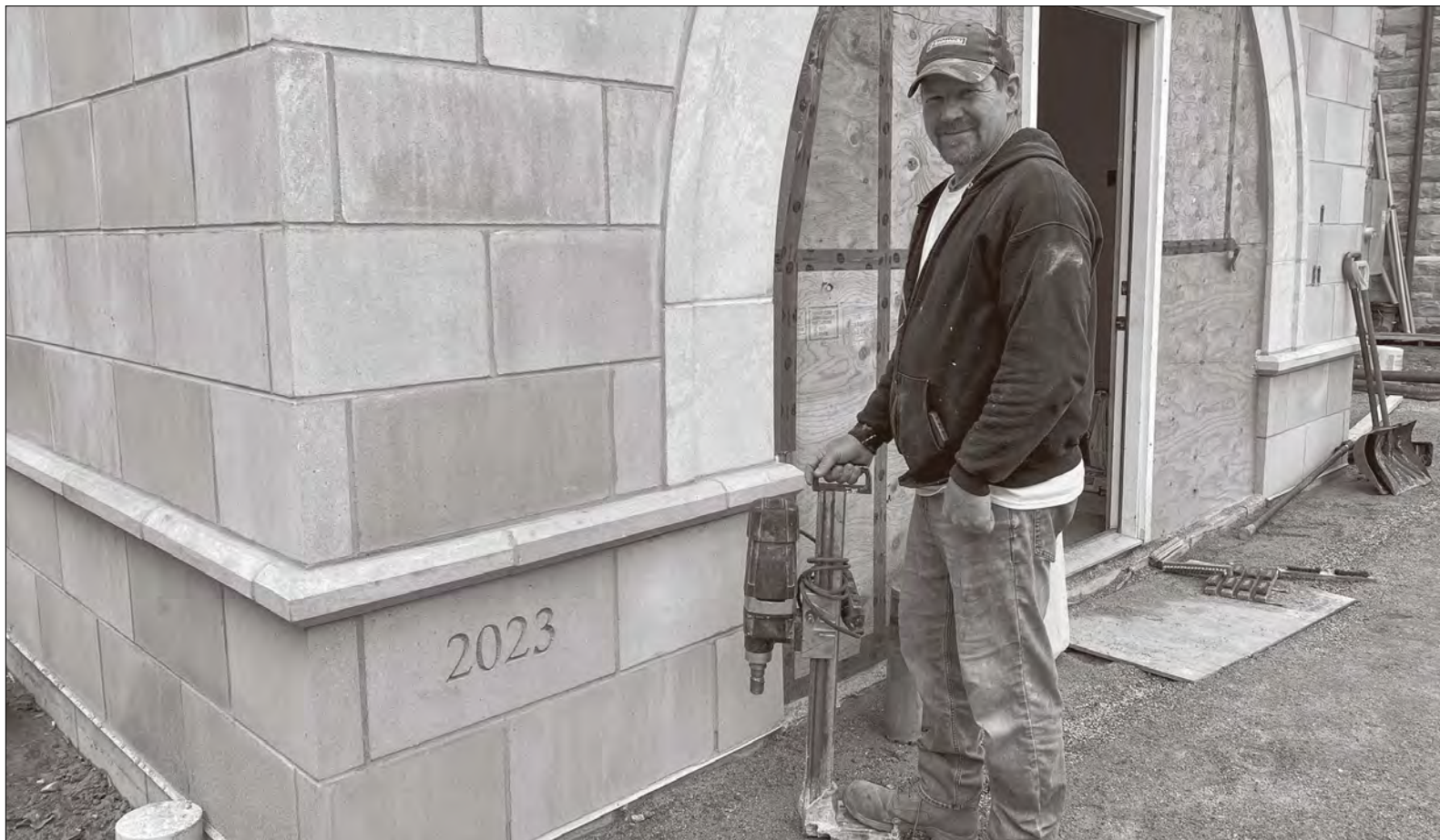
Troy DeBaise, Construction Supervisor from Kronenberger and Sons Restoration, outside the construction of the Hotchkiss Library of Sharon.
